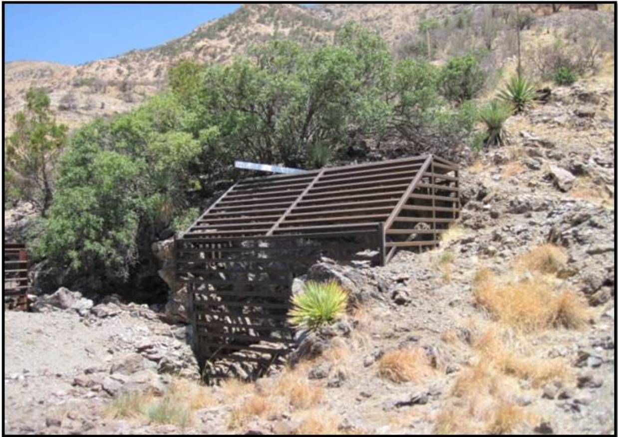
Figure 16. Final bat gate structure installed on a lesser long-nosed bat roost on the Coronado National Memorial.
